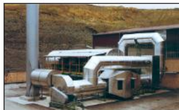
Modern brickworks with the flue gas cleaning systems all requirements of the German Technical Instructions (TA) Air
